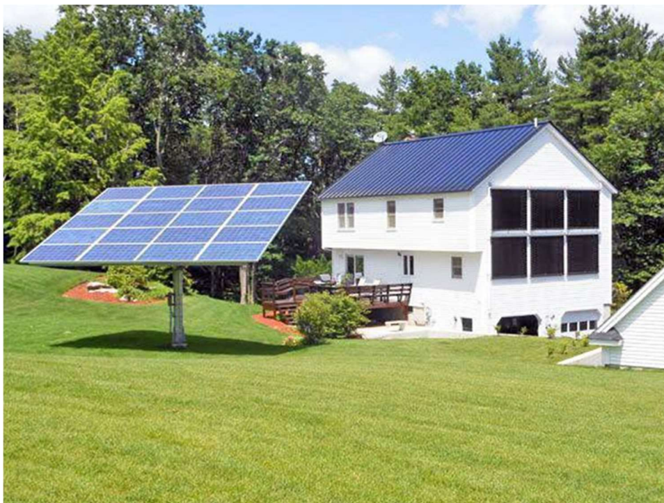
Tracker Mounted Residential System: Courtesy Revision Energy
