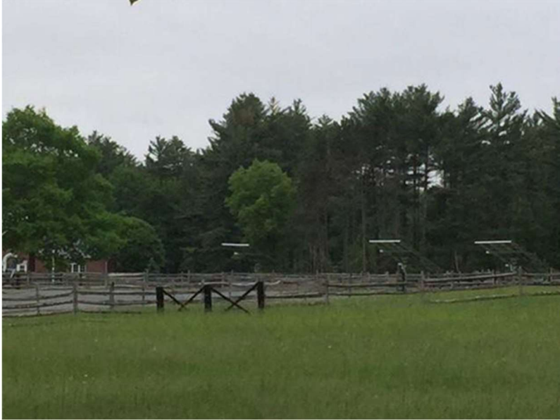
Pole-mounted system – agricultural site.
