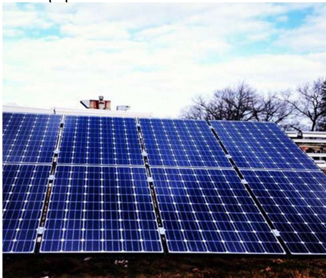
Completed installation showing gaps between panels
