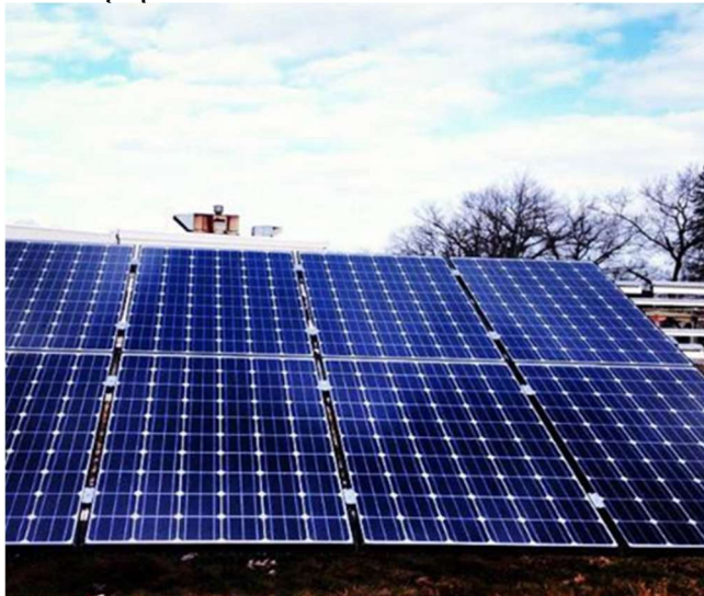
Completed installation showing gaps between panels
