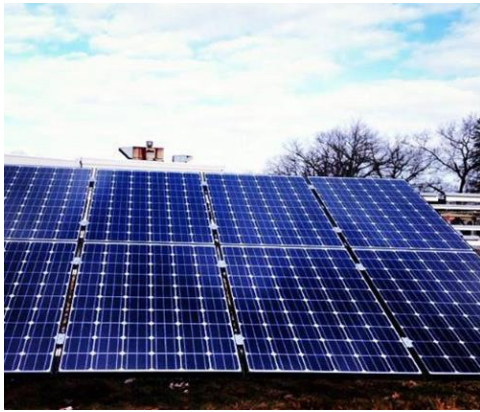
Completed installation showing gaps between panels
